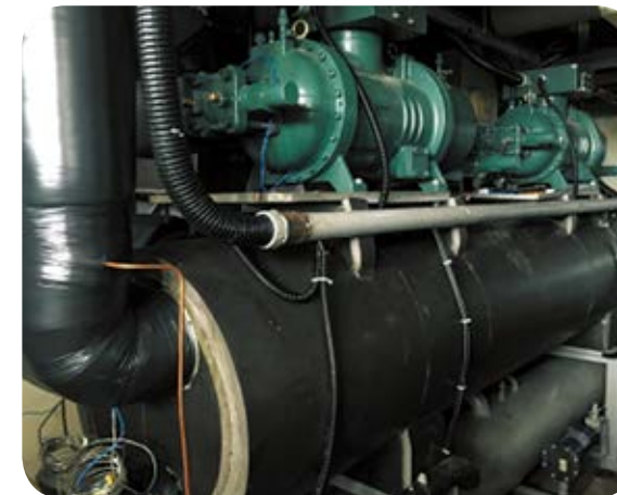
▲ Process backwater system of the Madou Bakery Plant.
