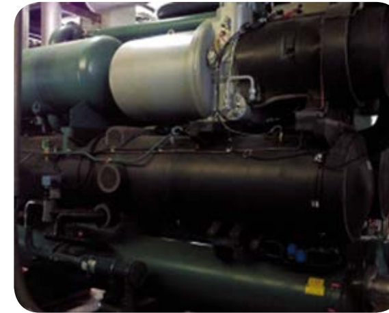
▲ The chiller system at the Yangmei Dairy Product Plant.
