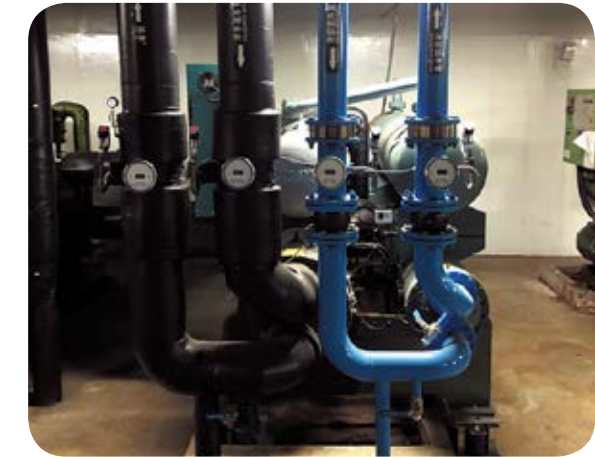
▲ Chiller of the dough freezing process of the Zhongli Bakery Plant.
