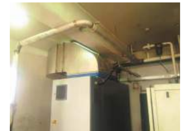
The actual view of the engine room for the air compressor at Madou Bread Factory
