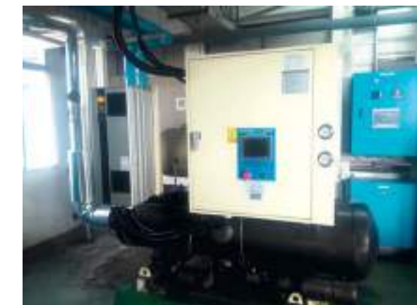
The actual view of the engine room for the juice processing water chiller at Drink I Plant of the Xinshi General Plant
