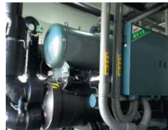
The actual view of the engine room for the water chiller at Yangmei dairy factory
