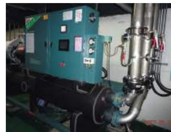
The actual view of the engine room for the water chiller at Ruifang Mineral Water Factory
