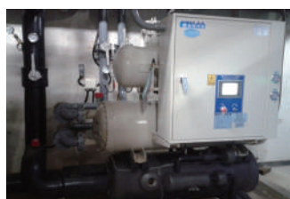
Figure. Super Air 55RT water chiller at the Taichung office building
