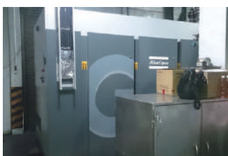
Figure. Air compressor unit at Yangmei General Factory
