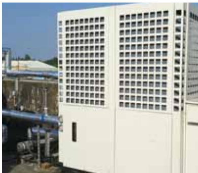
The main heat pump unit for the boiler water supply at Xinying Frozen Foods Factory
